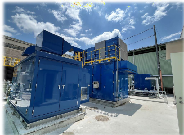
2MW gas turbine system (NEDO:JPN21020)
