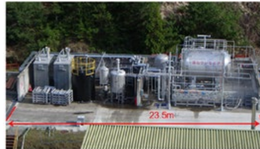
Large-scale ammonia supply system
