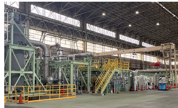
IHI's Large-scale Combustion Test facility (LCT)
