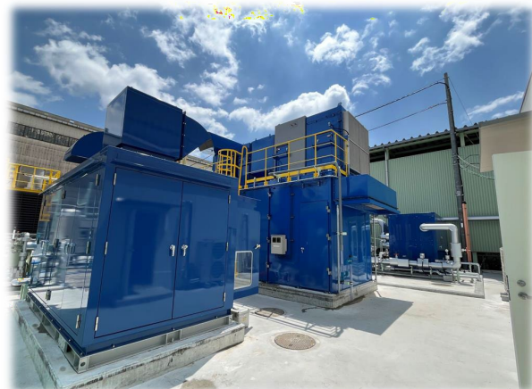
2MW gas turbine system (NEDO:JPN21020)
