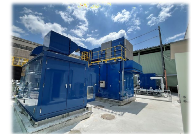
2MW gas turbine system (NEDO:JPN21020)
